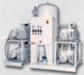
Mink Stack Mounted Quadruplex Vacuum System
